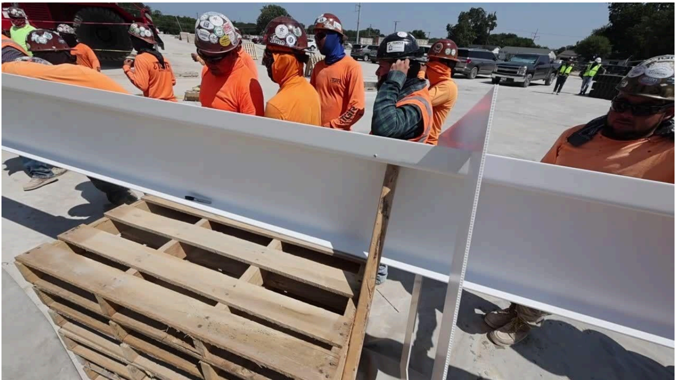
WATCH: Teachers sign the last steel beam before its installation Thursday, Aug. 8, 2024, at the new Kendrick Elementary School in Waco ISD.
